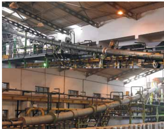
Figure 1 : 6 Nos. CCV (DRY CURE) LINES
